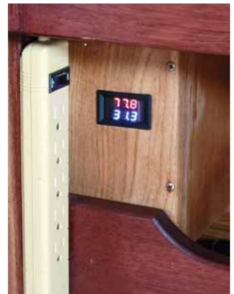
Installed panel and display unit
