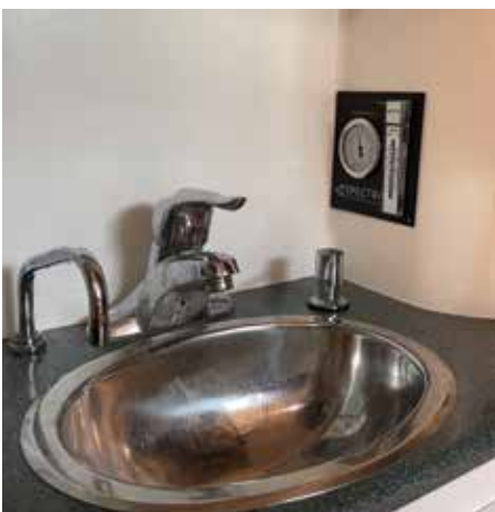
Gauge panel and discharge spout located in forward head.
