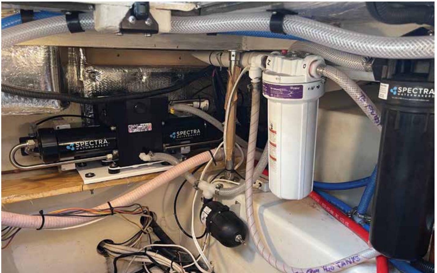
Clark pump and membrane located in bilge.
