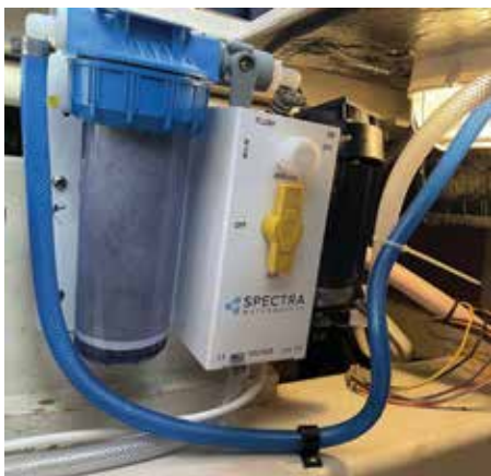
Feed pump module and charcoal filter located in bilge.
