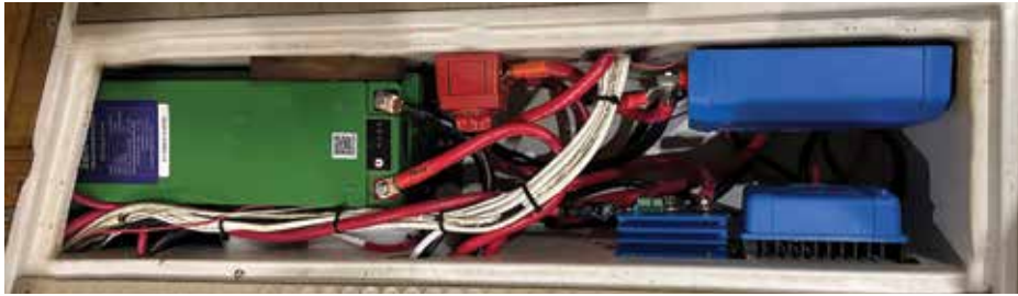
The stock battery box was used for 1 batter, a panel load switch, Victron Lynx Distribuion box, Victron Smart Battery Manager, and Victron DC to DC Charger for Starter Battery
