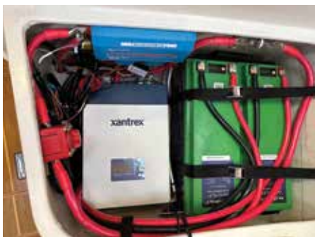
Storage area fore of sink contains two Kilovault 200Ah batteries, Xantrex Inverter Charger, Victron Lynx Battery Bus Bar, Battery Load Switch, two battery monitoring shunts and Class T fuse
