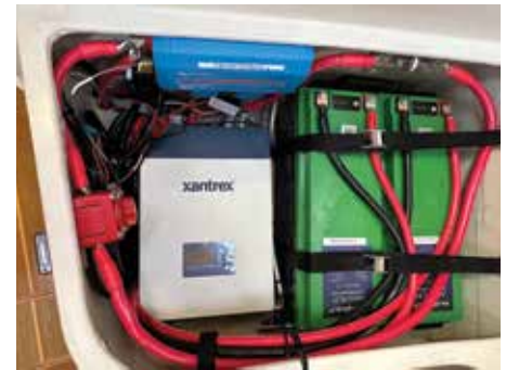
Storage area fore of sink contains two KiloValult 200Ah batteries, Xantrex Inverter Charger, Vic- tron Lynx Battery Bus Bar, Battery Load Switch, two battery monitoring shunts and Class T fuse.
