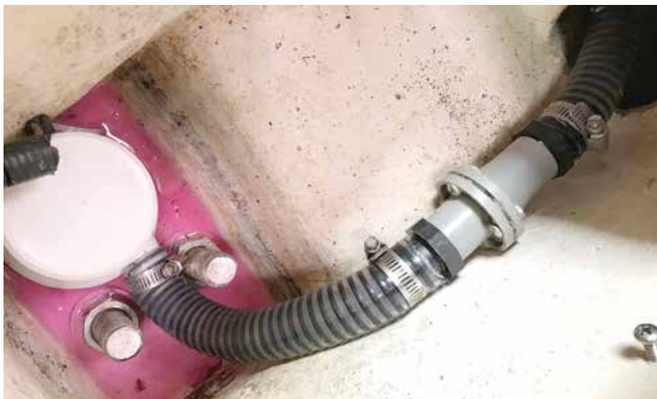
Electric bilge pump and hose running toward port settee with back flow valve
