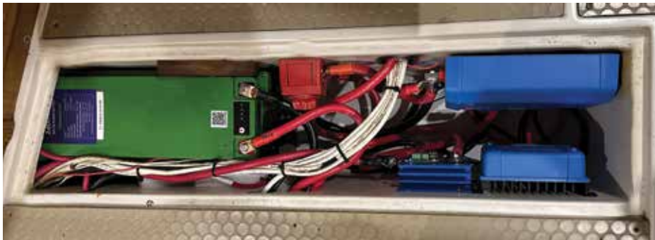
The stock battery box was used for 1 battery, a panel load switch, Victron Lynx Distribution box, Victron Smart Battery Manager, and Victron DC to DC Charger for Starter Battery.
