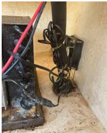
Compressor/condenser and fan in locker
