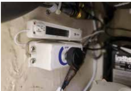
Thermostat control and freezer monitor
