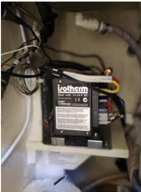
Isotherm Comp on shelf under galley sink
