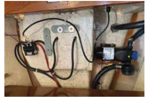
Wiring for windlass
