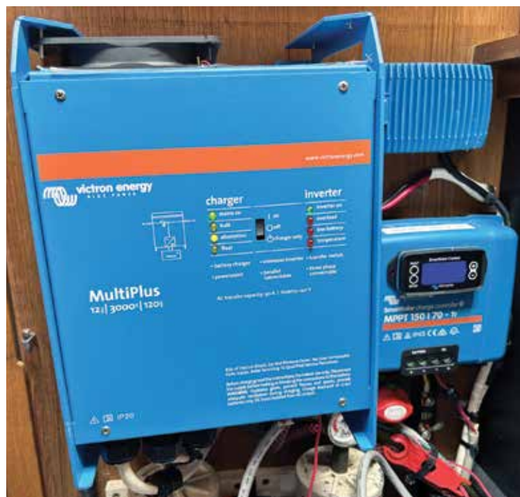
Inverter/Charger, solar MPPT controller
