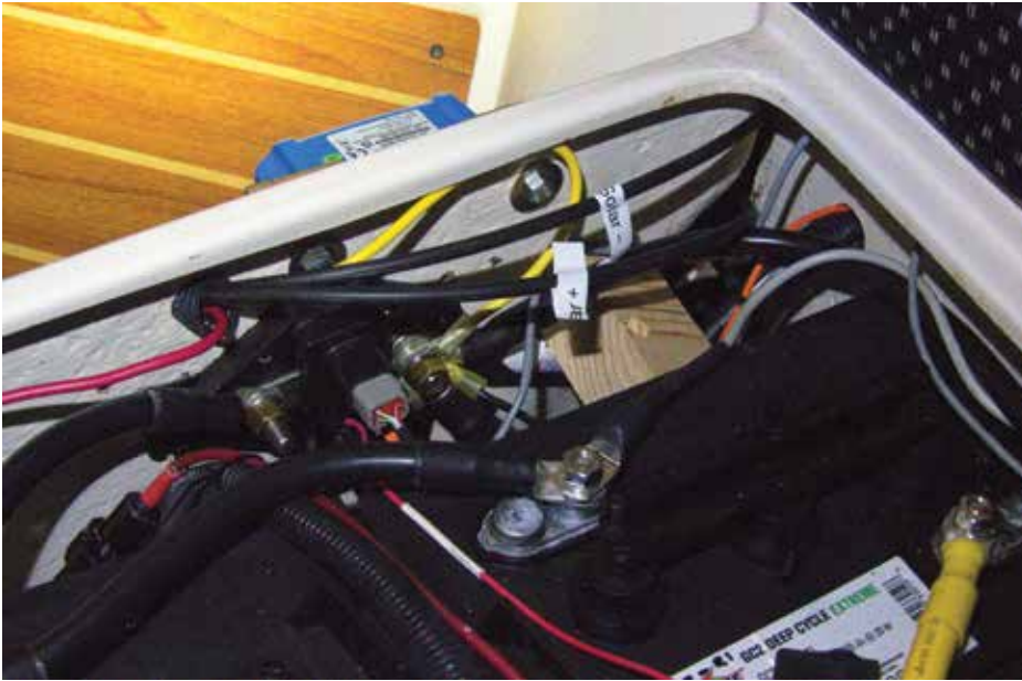
Battery compartment with solar controller top in blue, seen under nav station. Note labeled solar panel wires.
